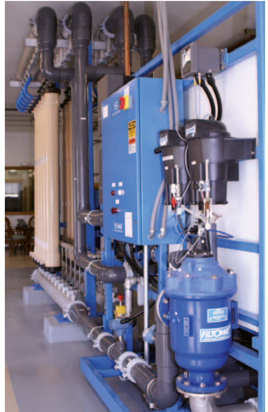
Lakeview's Pall Aria systems are compact and expandable to meet future demand growth.
