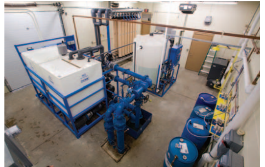
The Village of Groton solved its groundwater challenges with a Pall Aria microfiltration membrane system.
