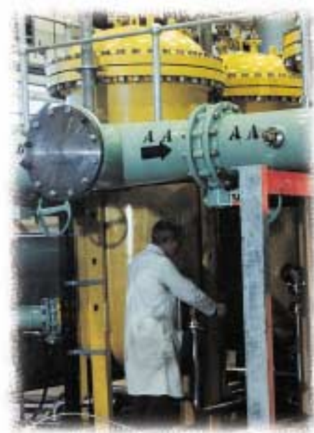
Pall blowback filter system in operation.
