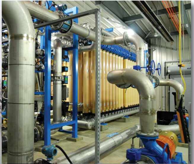
The system's pipes, pumps and filtration modules.
